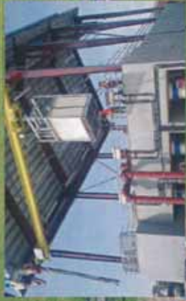
Membrane Reactor Basins
