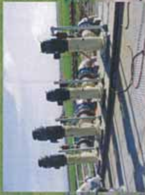
Effluent Pump Station
