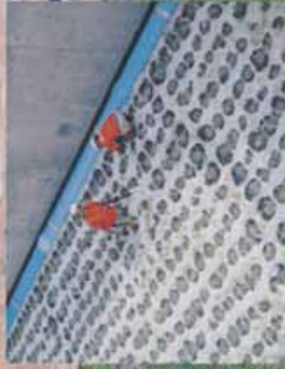
Aeration Basin Membrane Diffusers
