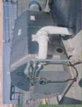
Headworks - Drum Screens
